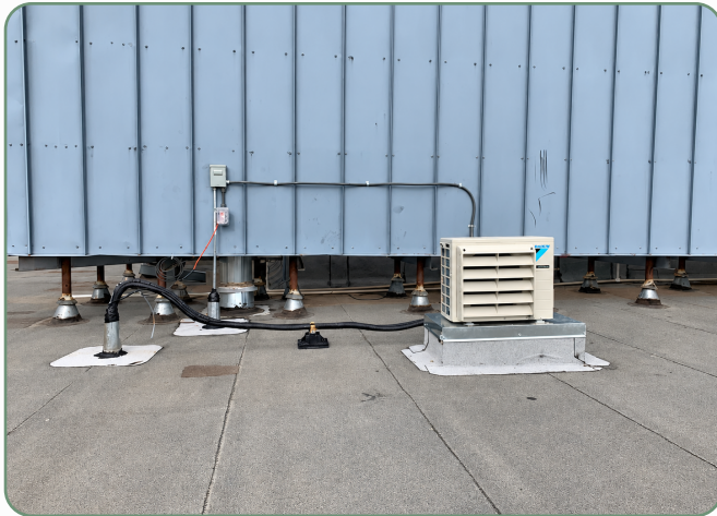
SUPPLEMENTAL COOLING | COMPLETED
